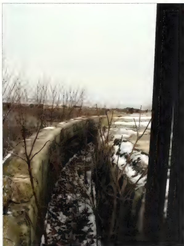
Figure 3.34. View looking east at the chemin de ronde , Battery Potter. The chemin de ronde is presently a collection area for leaf litter and debris that supports the growth of woody vegetation (Olmsted Center, January 2009).
